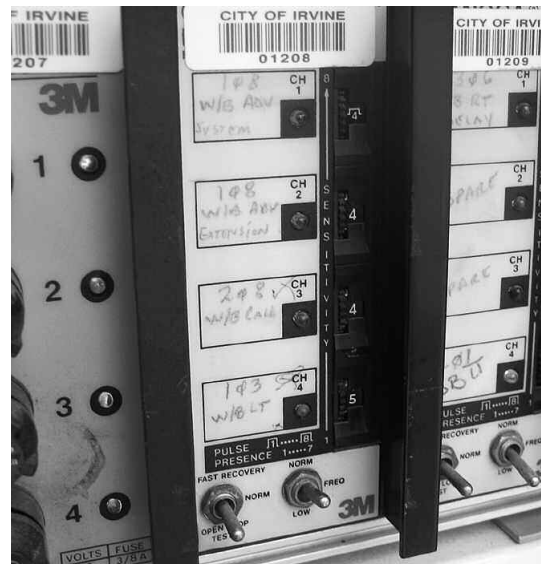
Inside the loop detectors' control box: Each light turns on when a vehicle is detected. The bottom sensor, for a left turn signal, is set to be slightly more sensitive because of a weaker field.
